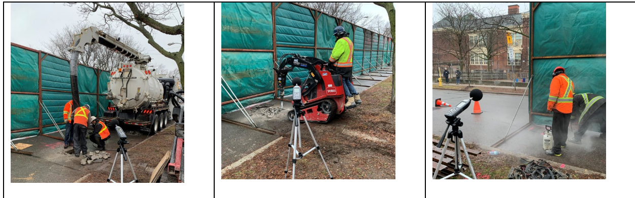
Figure 4-3 Temporary Noise Barrier
